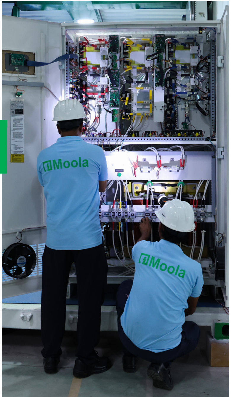
Moola personnel performing maintenance duties on a BESS Unit
